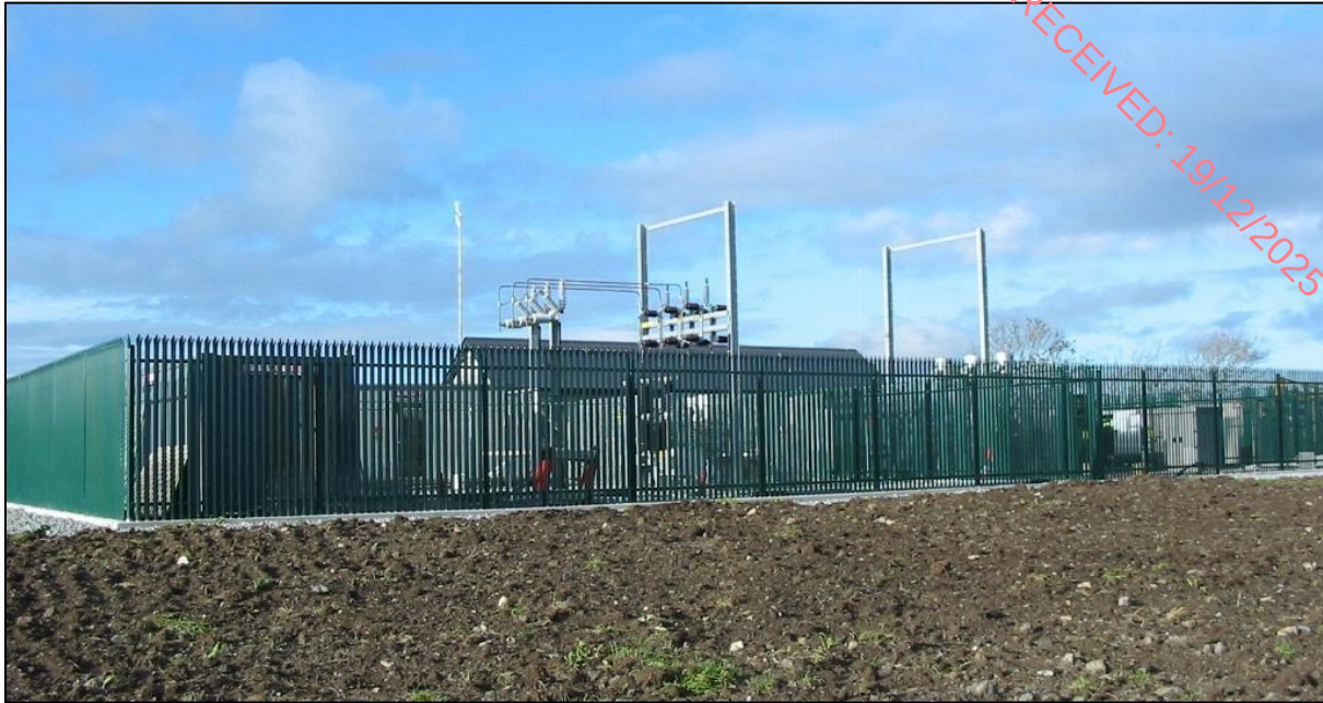
Figure 4-6: Example of a Substation Compound
